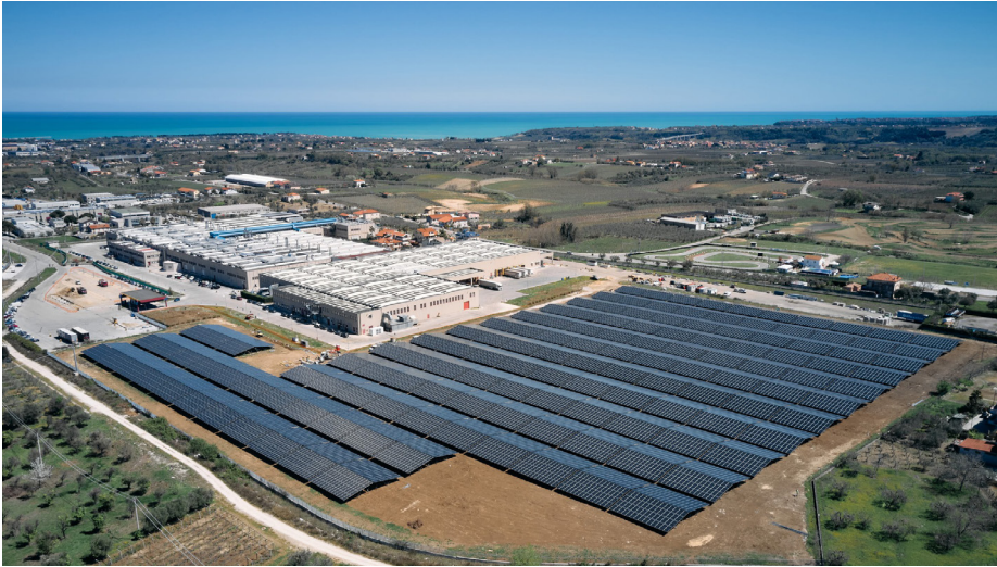
CHART 13 – PHOTOVOLTAIC SYSTEM REALIZED IN ORTONA IN 2022
